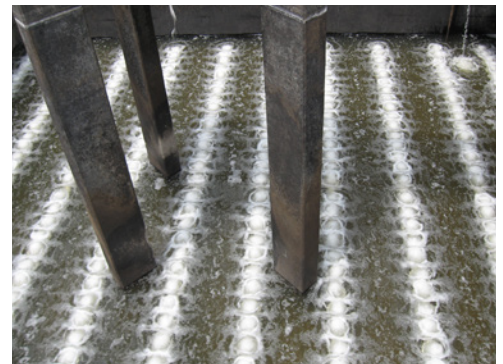
Quantaer Fine Bubble Aeration System
