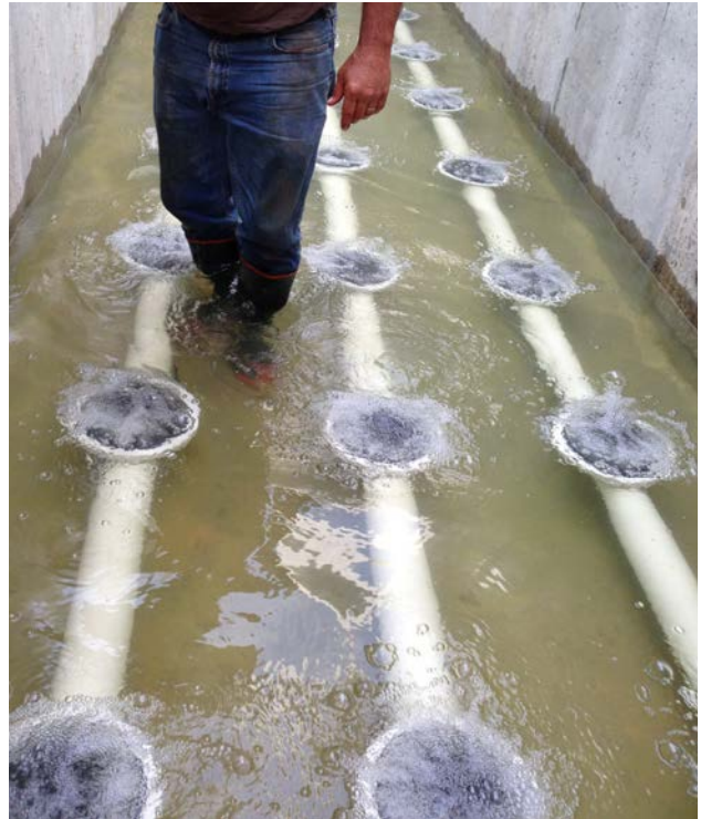
Fine Bubble Membrane Disc Diffuser Grid Integrated below the Fixed Media Structure
