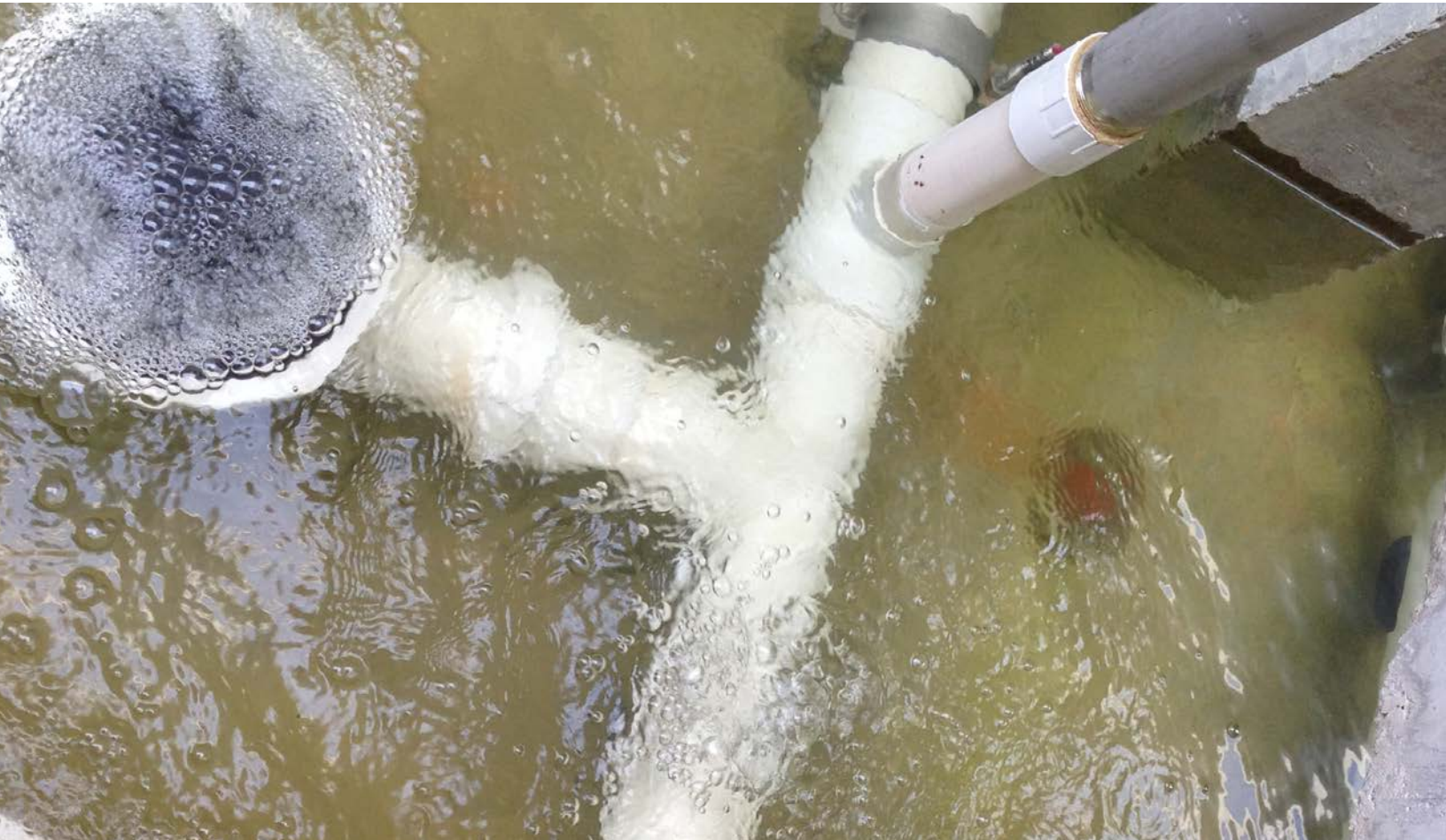
Fine Bubble Membrane Disc Diffuser Used to Deliver Oxygen Necessary for Organic Treatment and Scour Media
