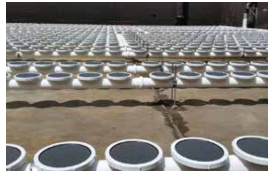
Quantaer Aeration Delivery System
