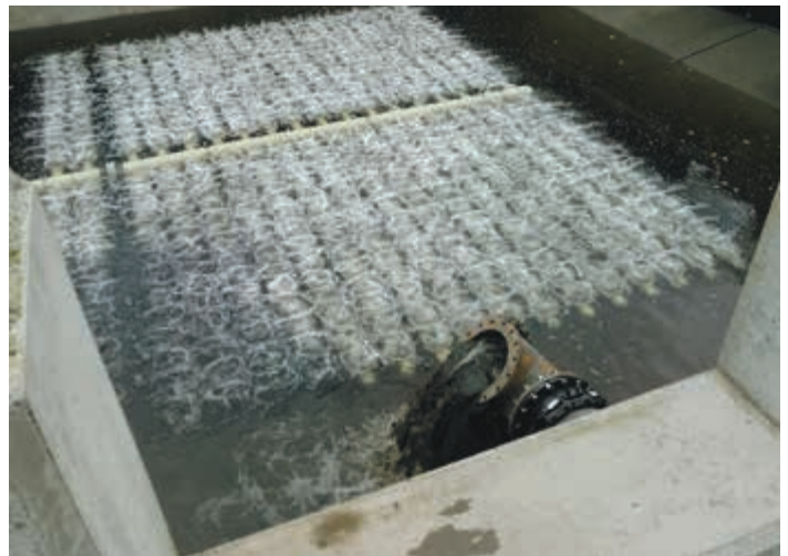
Fine Bubble Aeration System in Operation
