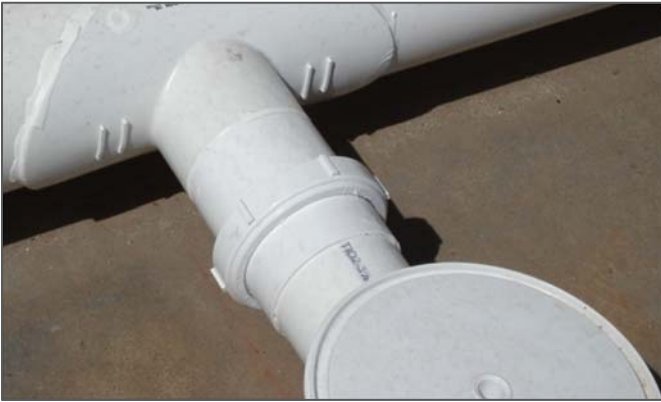
Air Distributor Connected to Air Manifold
