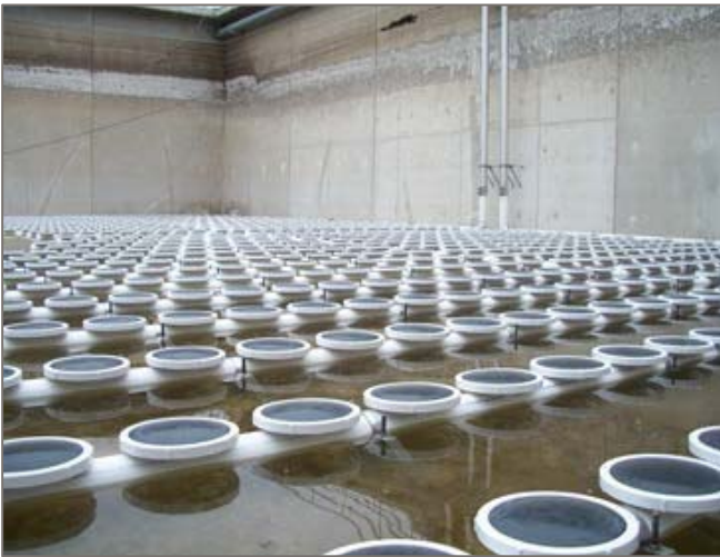
Quantaer Fine Bubble Aeration System Installation
