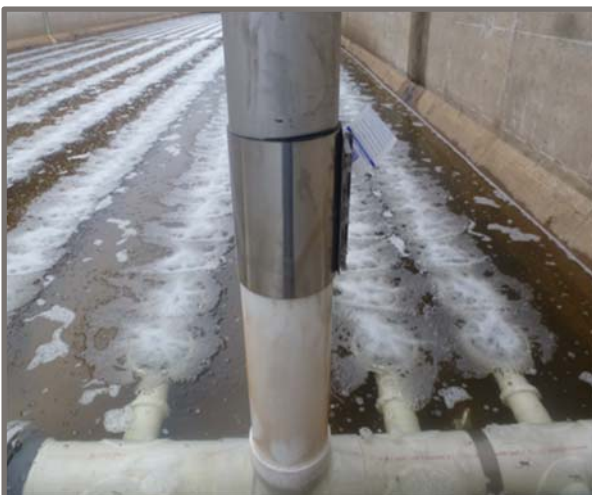
Drop Pipe and Air Manifold Connection
